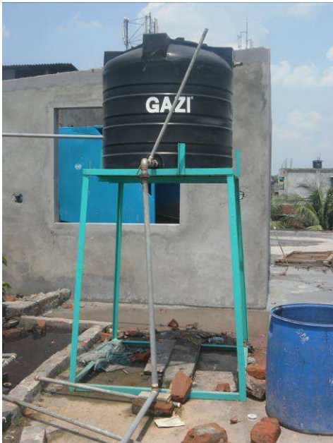
Figure 2. Inlet water tank to solar collector
