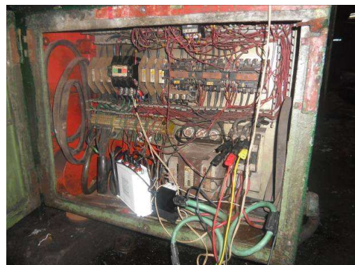
Figure 10. Capacitor's battery and contactor installation in the electrical and control board of the setting machine
