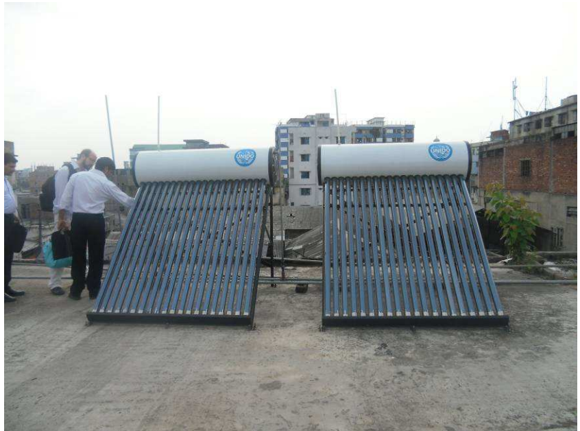
Figure 3. Thermosiphon solar hot water collectors
