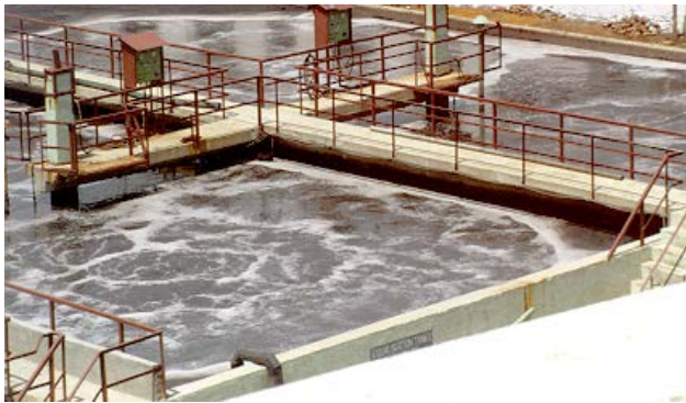
Fig 2. : Ejector aerator in the equalization tank
